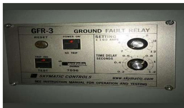
Gambar 2. 18 Proteksi Groundfault Relay (OCG)
