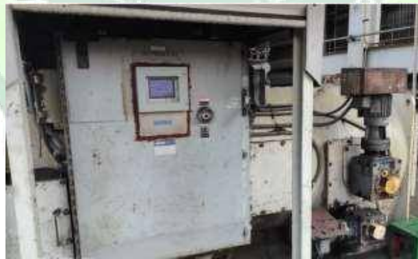
Gambar 4.15 Motor coal feeder PLTU Tanjung Jati B Unit 1 & 2
