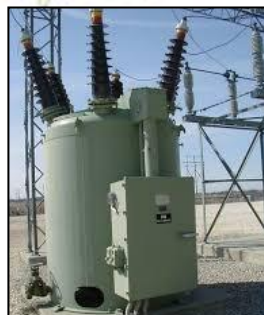
Gambar 2.16 OCB ( Oil Circuit Breaker )
